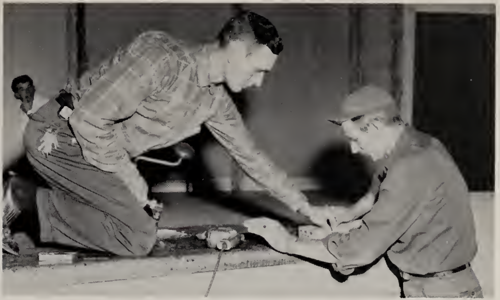
Mr. Durbin, Supervisor of Buildings and Grounds, is shown here with Bill Shook as they do some repair work on the stage.
